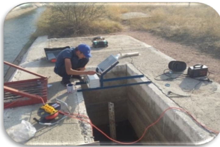
Figure 11. Installation of the DUV 2/0,005-10 device on the surface of the stilling well.
